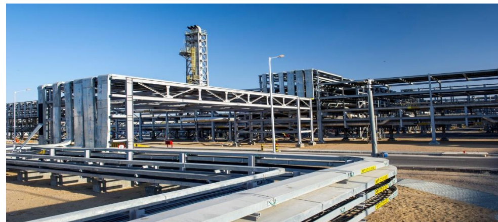
Rajasthan: Mangala Processing Terminal
