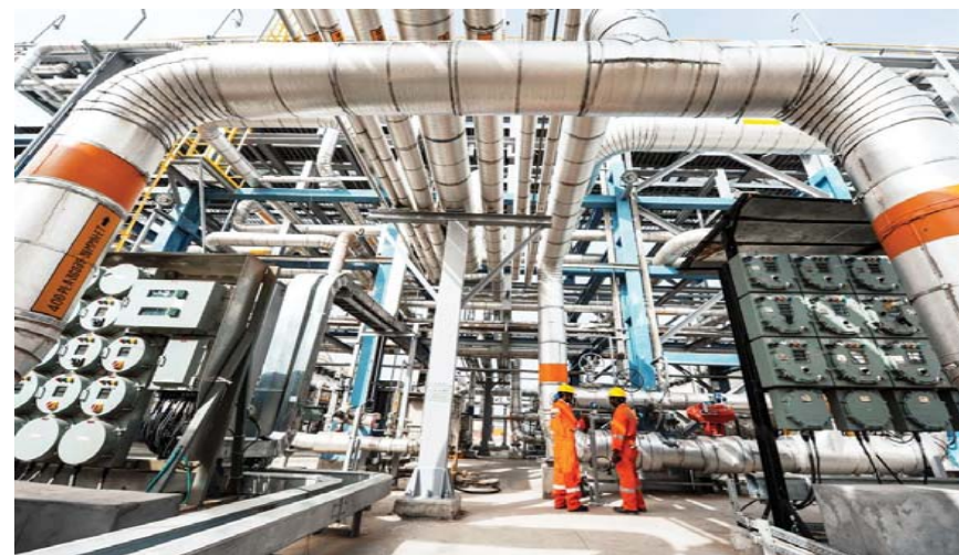
Rajasthan: Crude Oil Processing Facility
