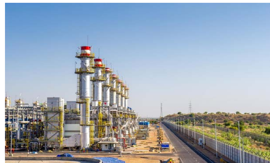
Rajasthan: Captive Power Plant - Steam Generation
