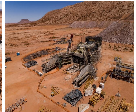
ROM - Primary Crushing
