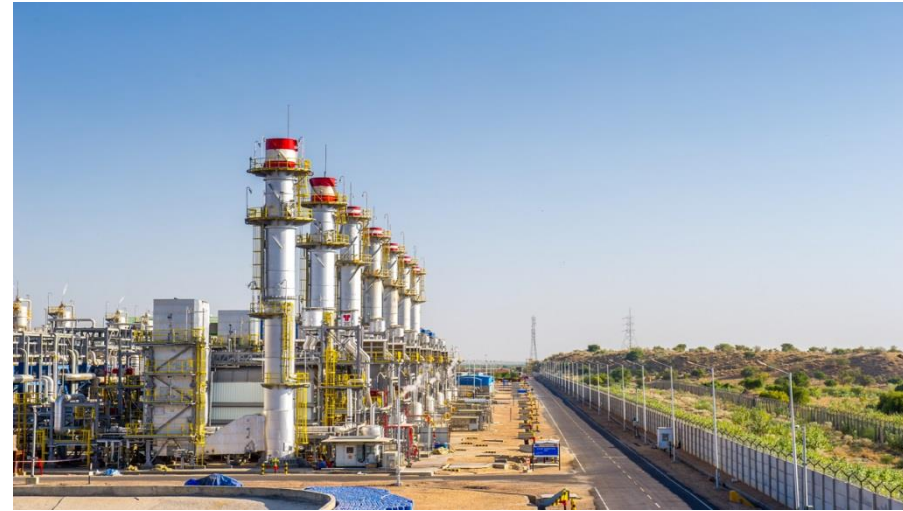
Rajasthan: Steam Turbine Generators at Mangala
