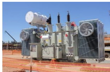
Transformer installed on site
