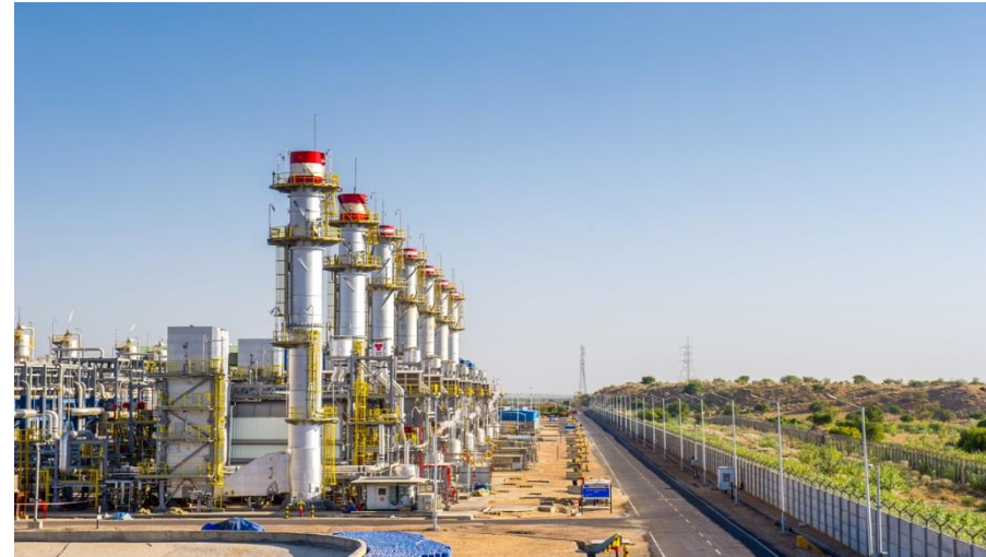
Rajasthan: Steam Turbine Generators at Mangala
