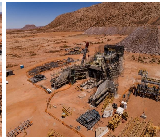
ROM - Primary Crushing
