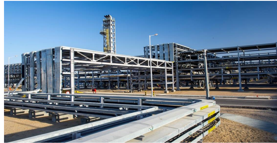
Rajasthan: Mangala Processing Terminal
