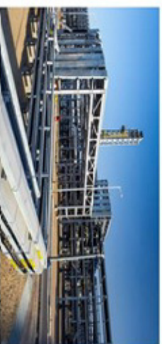
Mangala Processing Terminal
