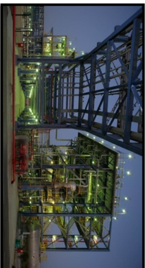
Rajasthan: Raageshwari Gas Terminal
