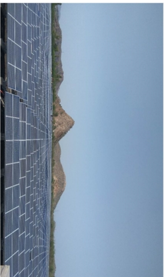
Hindustan Zinc Limited solar panels
