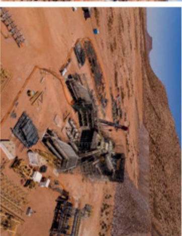
ROM - Primary Crushing
