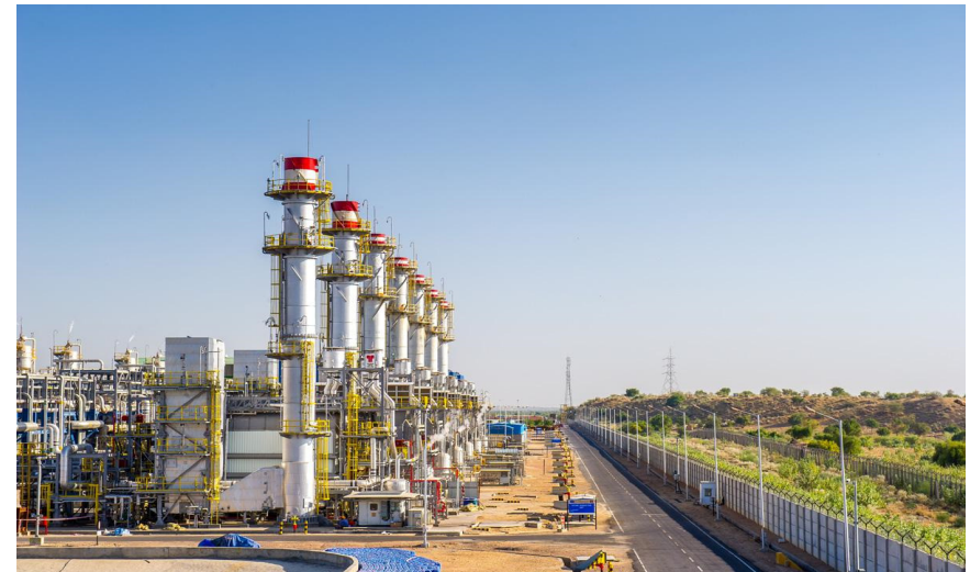
Rajasthan: Captive Power Plant - Steam Generation
