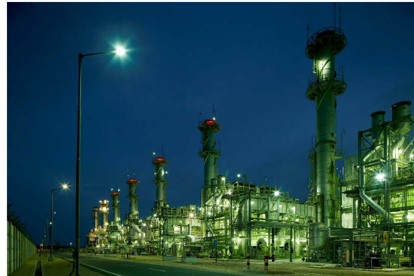
Rajasthan: Mangala Processing Terminal
