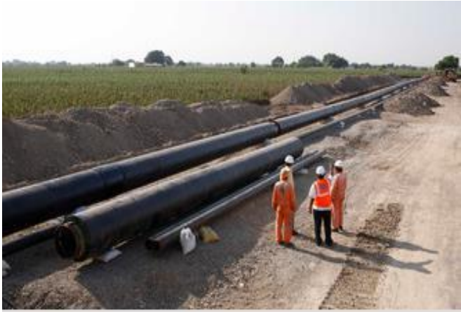
Worlds Largest continuously heated pipeline
