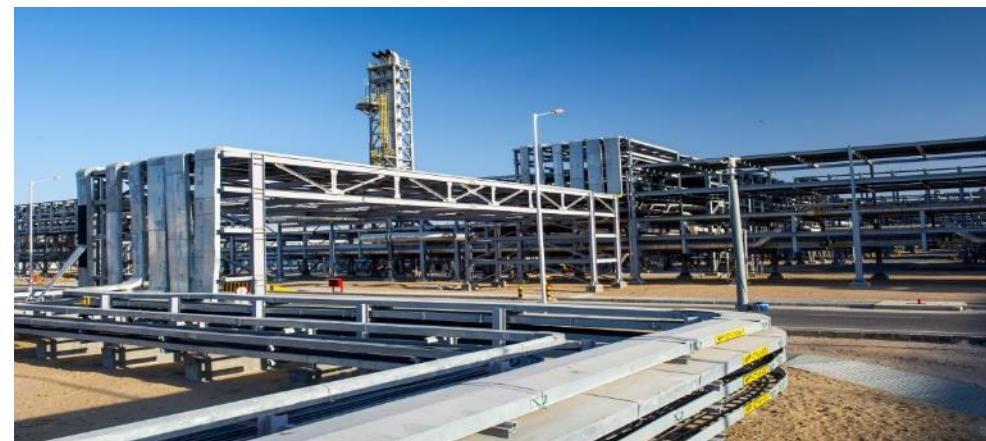
Rajasthan: Mangala Processing Terminal
