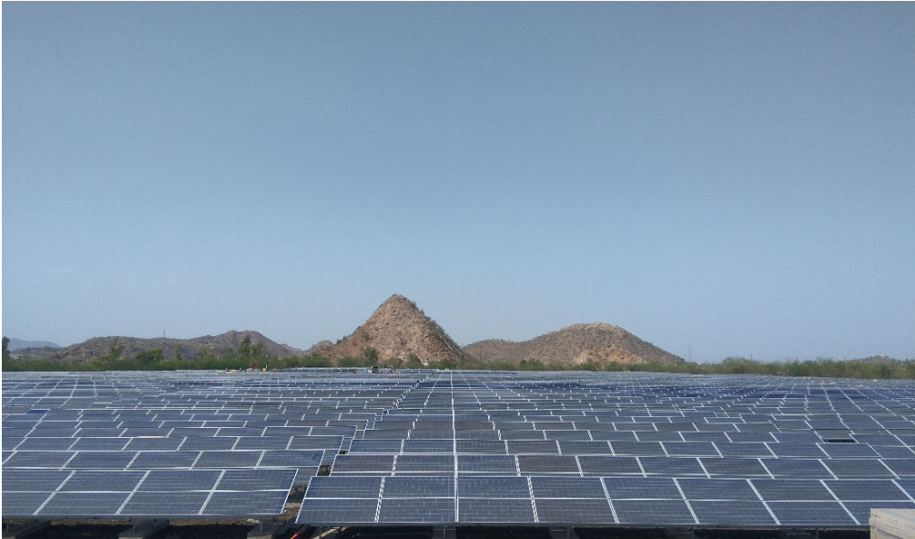
Hindustan Zinc Limited Solar panels
