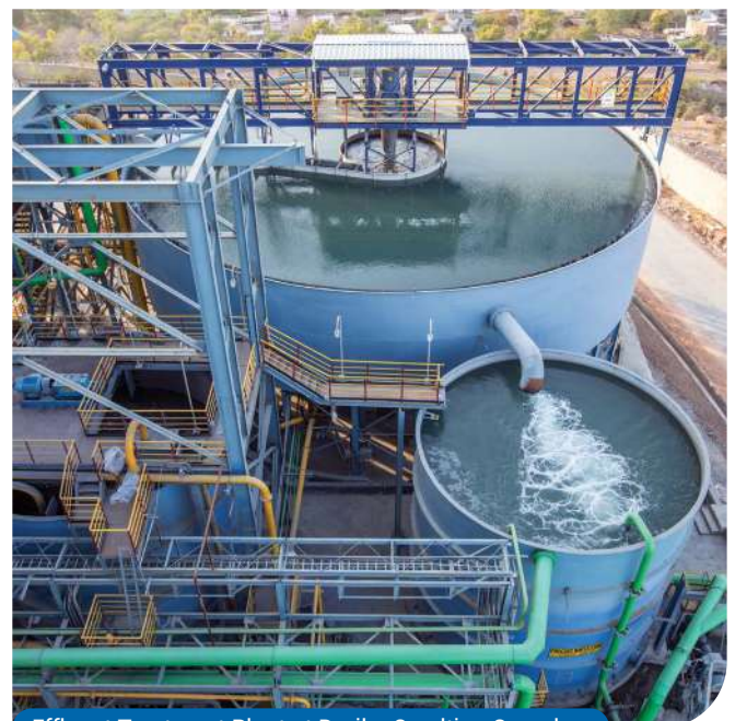
Effluent Treatment Plant at Dariba Smelting Complex
