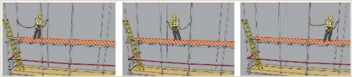
To traverse, double lanyards are used to remain continually attached, ideally to inner standard or ledgers
