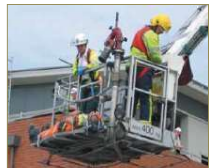
Figure 58: Scaffolder working without a fully-boarded platform
