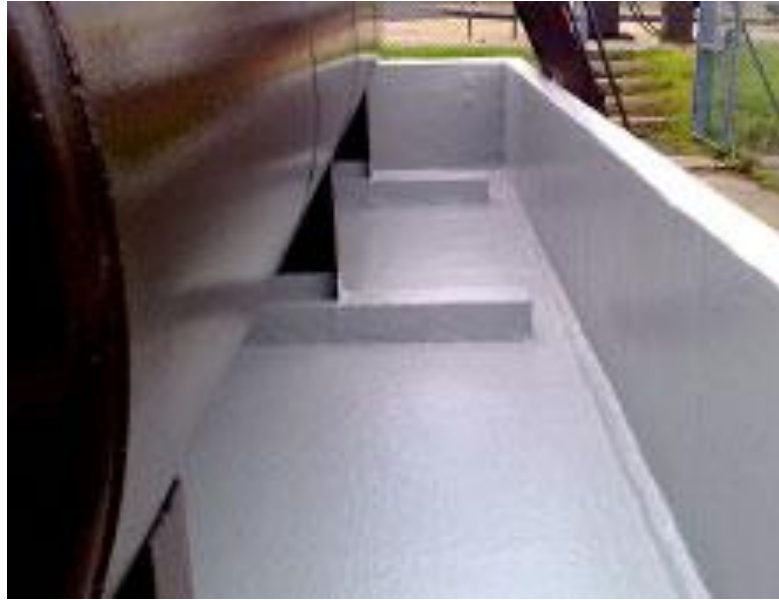
Example of a bulk storage tank with secondary containment
